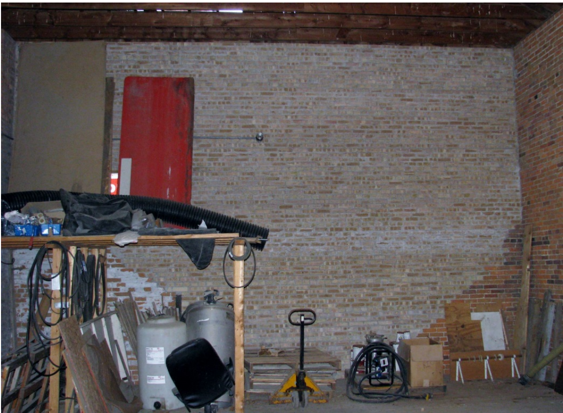
South wall – Non-historic Brick Condition, Interior
