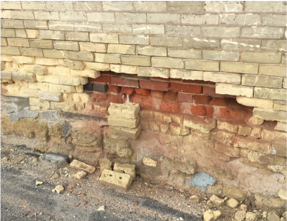
Water damage and degraded masonry
